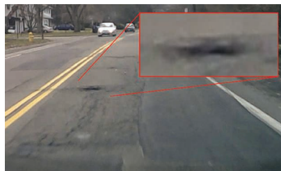
FIG2 A pothole in the road.
